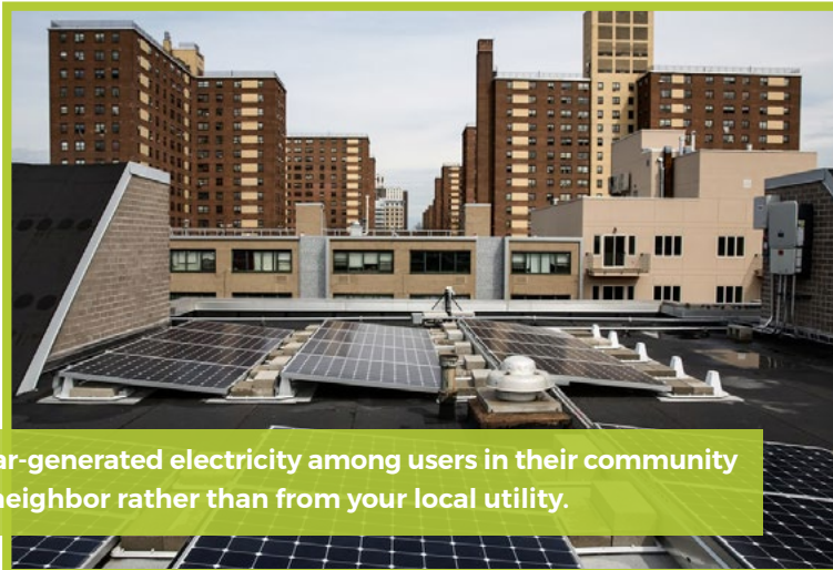
Rooftop solar at Marcus Garvey Village in Brooklyn. Photograph: Demand Energy
